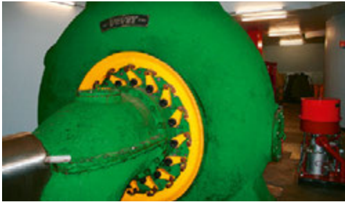
Isolation an Turbine
