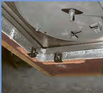
Asbesttextil in Kochherd
