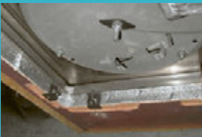
Asbesttextil in Kochherd
